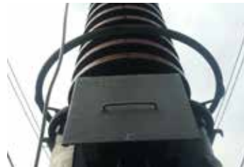
Inspection boxes protected from corrosion
